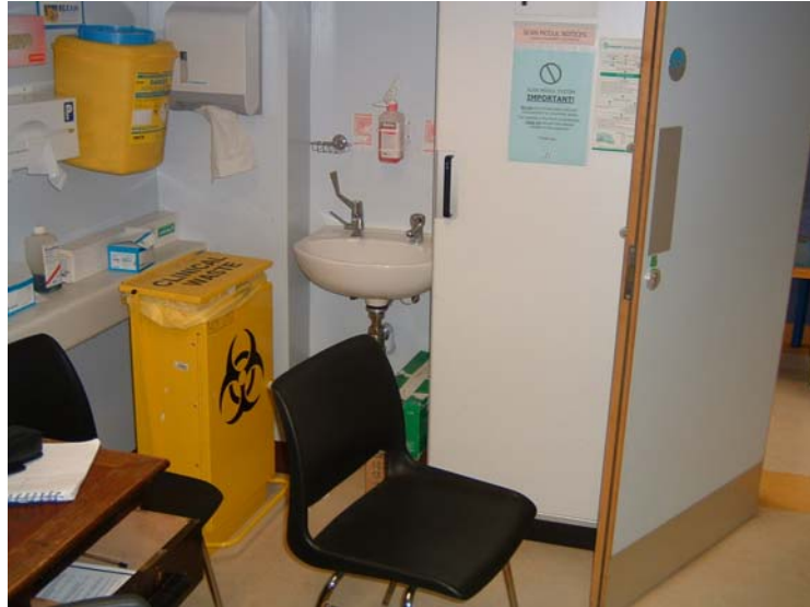
FIG. 15: Press, hand sink and open drawer (bottom left) in treatment room
